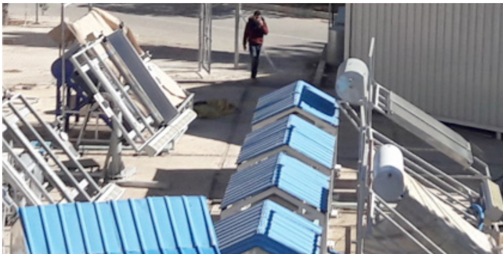
Figure 22: NERC Solar Thermal test lab in Jordan
