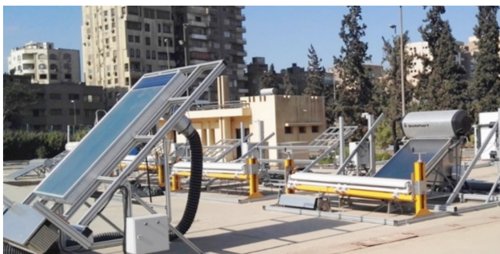
Figure 19: NREA Solar Water/Air Heaters Test Lab in Egypt
