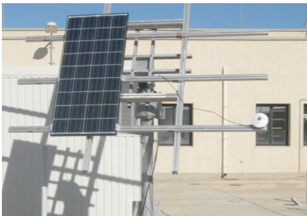
Figure 30: CSERS Solar PV Conversion Lab
